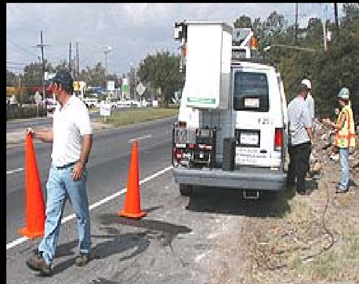
Photo courtesy of the U.S. Army Corp of Engineers. This picture shows actual disaster site work conditions and may not illustrate proper safety and health procedures.
